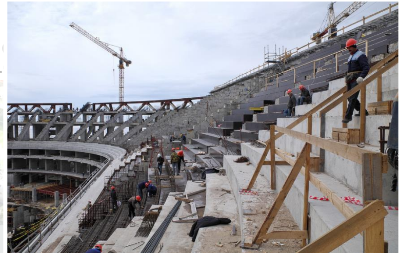
Case in slab joints
